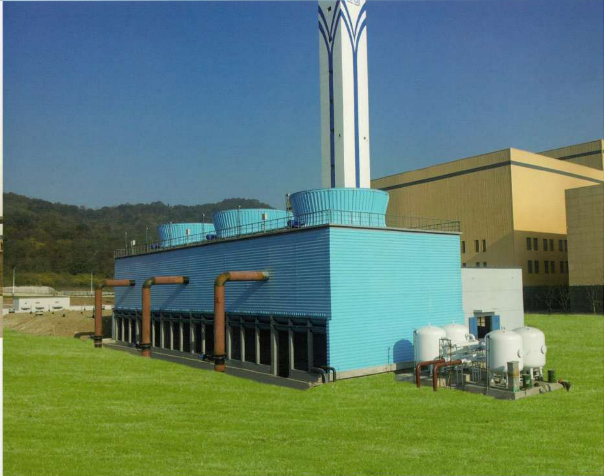
南京市江北静脉产业园垃圾电厂 Nanjing Jiangbei Industrial Park Intravenous Garbage Power Plant SHN-3500×3型冷却塔
